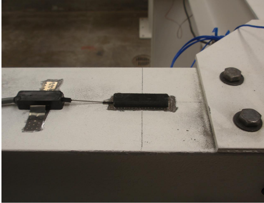
Figure 3.16: 350 Ohm weldable strain gage installed on grid model structure. Photo taken by Jason Herrman, Fall 2010 Engineering Research Center
