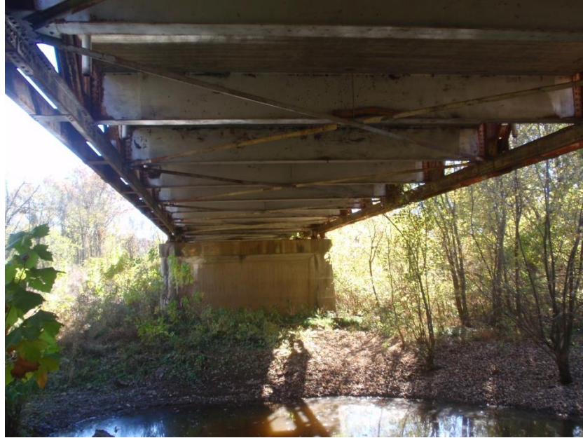
Figure 4.5: Baptist Ford Bridge - View from Underside Photo taken by Jeremy Rawn, Fall 2010 Fayetteville, Arkansas
