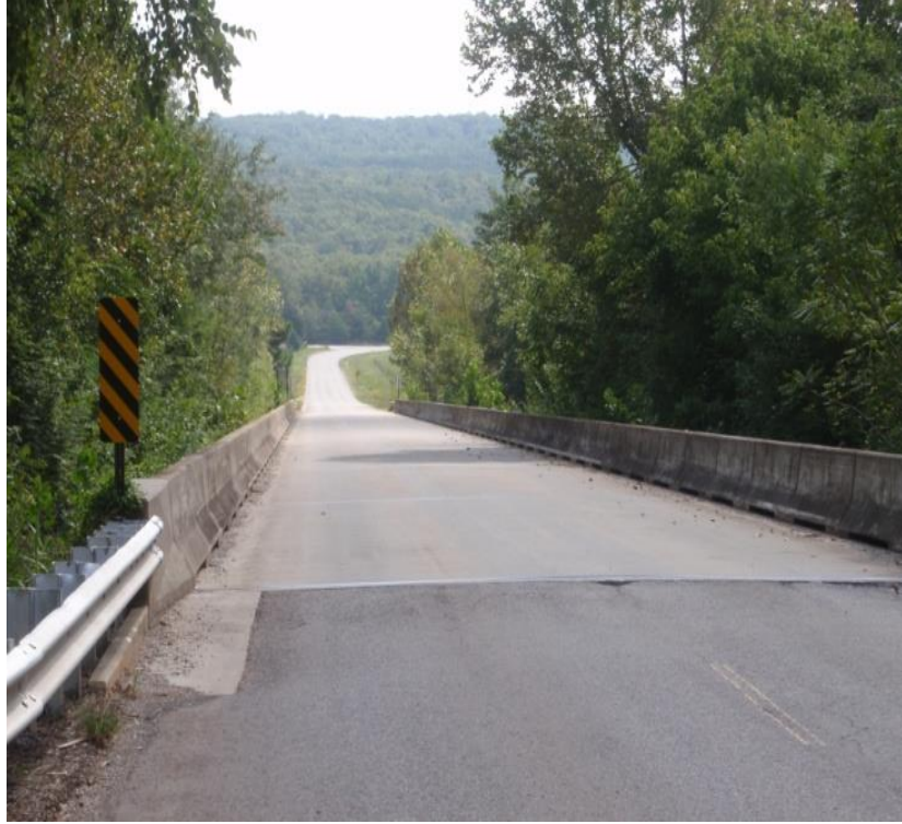
Figure 4.1: Hancil "Tiny" Hartbarger Bridge - concrete deck on multi-beam bridge. Photo taken by Jeremy Rawn, Fall 2010 Fayetteville, Arkansas
